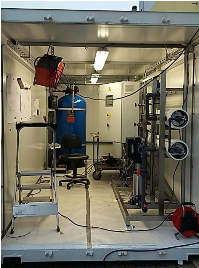
Figure 2. Water processing unit, outside (up) and inside (down)
